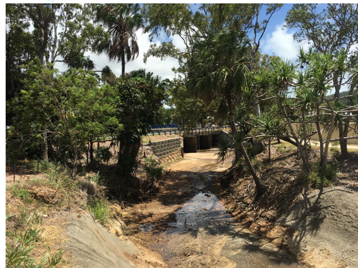
Figure 15 - This part of Fig Tree Creek is an immediate priority
