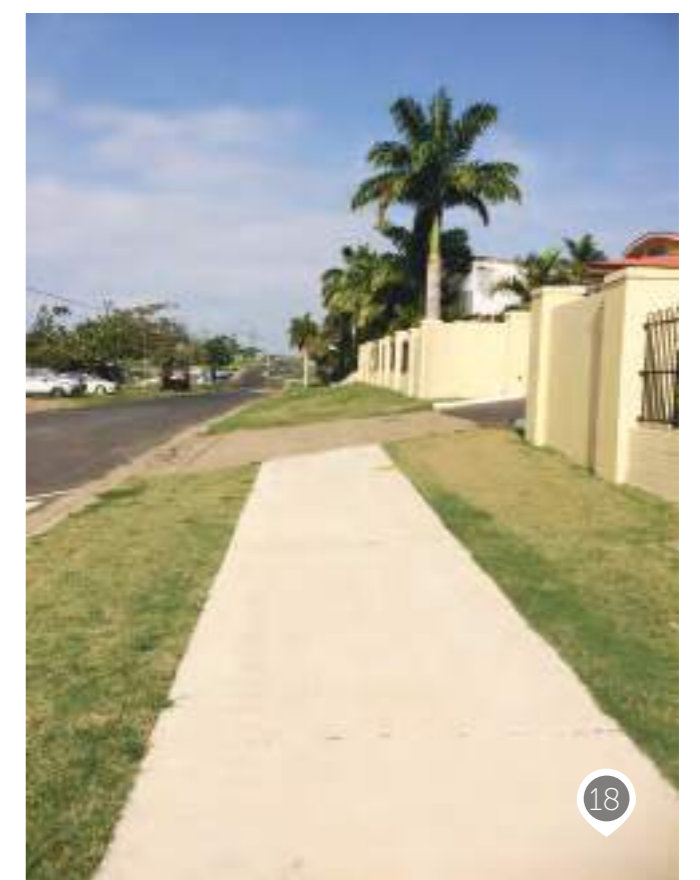
Photo 18 Incomplete footpath along Queen Street
