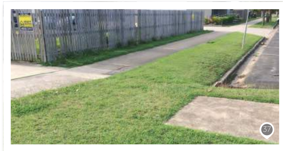
Photos 37-38 Incomplete footpath at intersection of John and Arthur. Footpath – road interface is not universal accessible.
