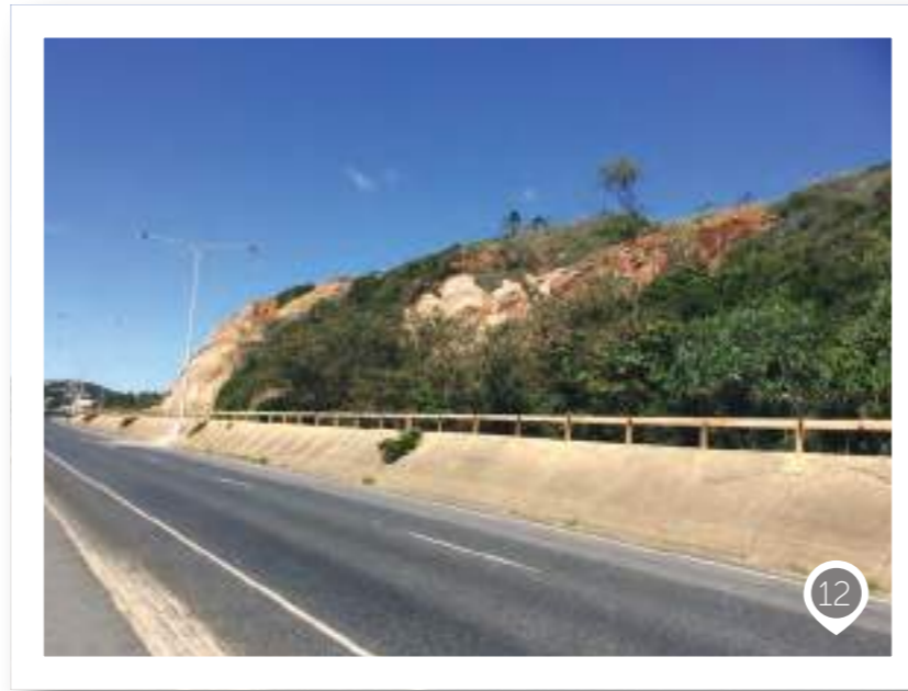
Photo 12 Sloped concrete centre median illustrating planter hole impact
