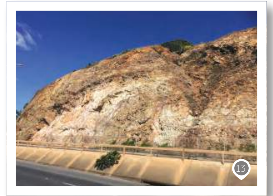
Photo 13 Bluff on west verge of Farnborough Road immediately prior to Yeppoon entrance
