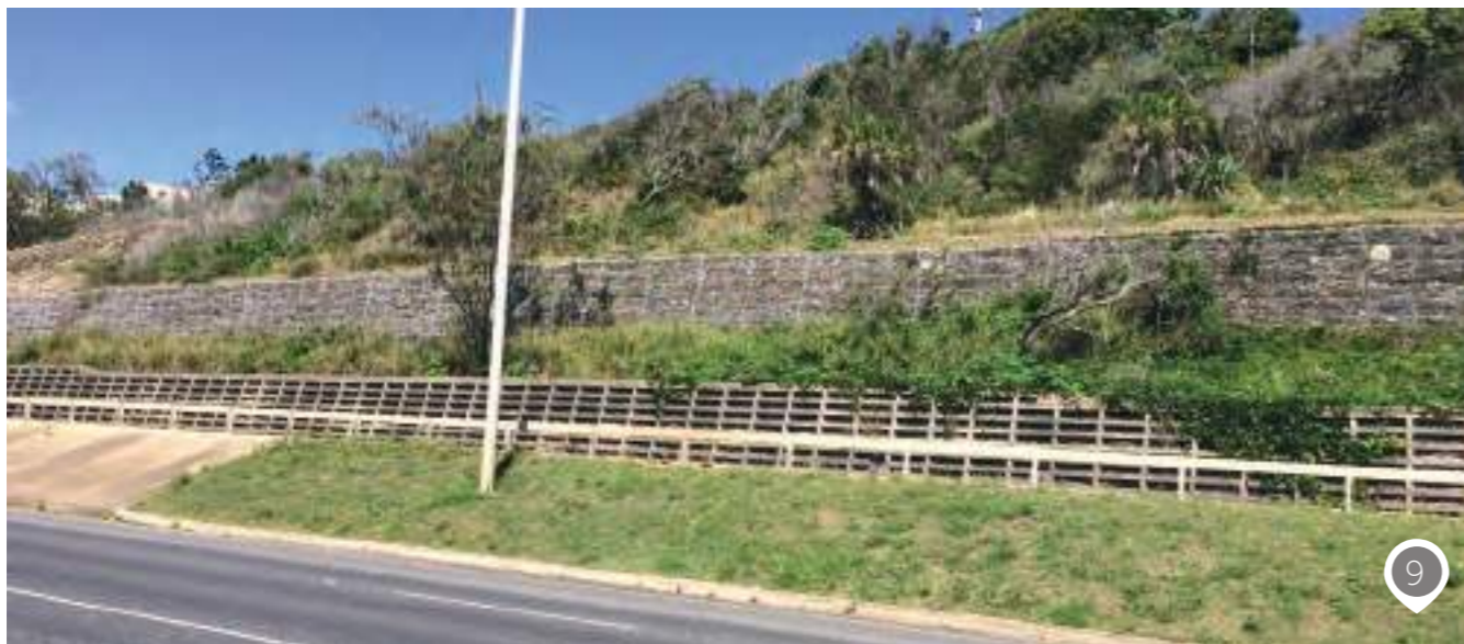
Photo 9 Centre median and revetment walls on west verge of Farnborough approaching Yeppoon
