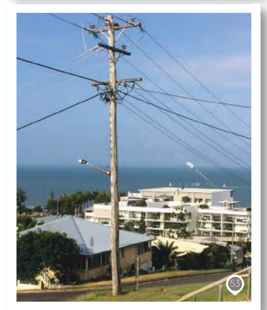
Photos 52,5 3 Ergon poles John/Hill Street and Queen/Arthur Street
