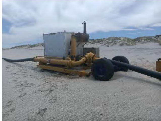
Figure 6-6 Pipeline booster pumping station
