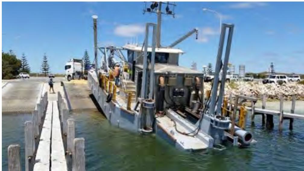
Figure 6-9 Launching of a small CSD off a semi-trailer, at a commercial boat ramp
