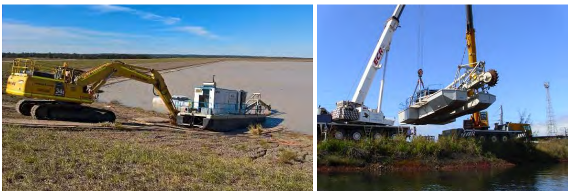
Figure 6-14 Left: Mini CSD pushed into the waterway with a medium size excavator; Right: CSD launching with a two-crane lift
