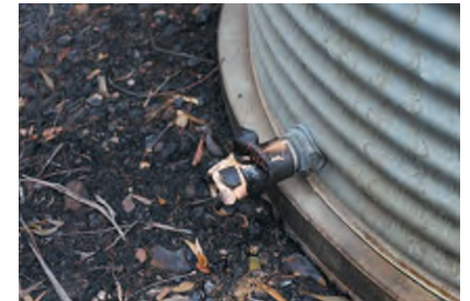
Combustible pipe fitting melted. Source: CSIRO
