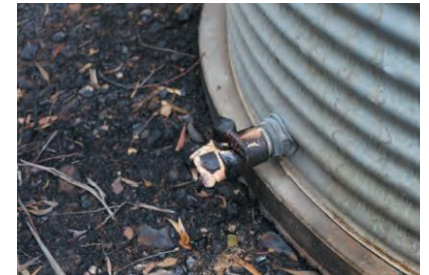
Combustible pipe fitting melted. Source: CSIRO
