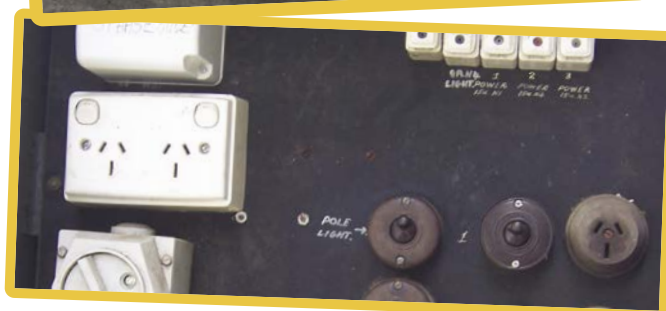
Zelemite backing board to an external switchboard
