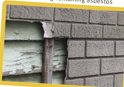
External cladding containing asbestos
