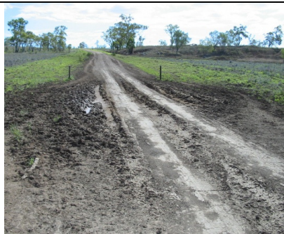
No Gravel Pavement
