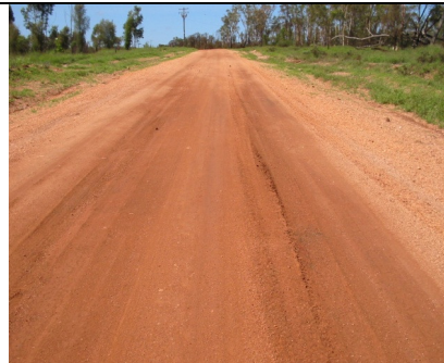
Poor Gravel Pavement
